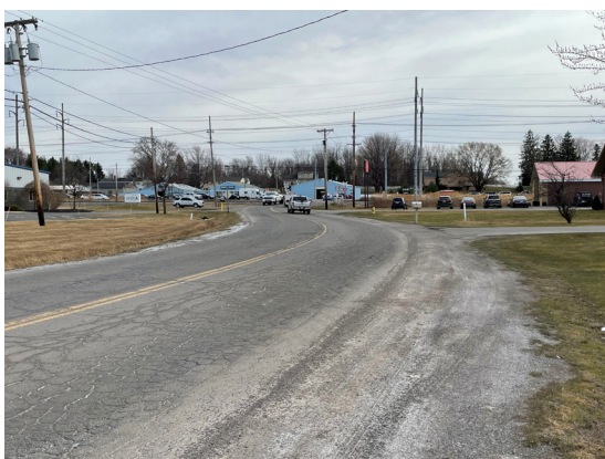
Dean Pkwy typical pavement condition
