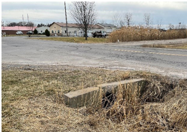
Damaged headwall along Dean Parkway
