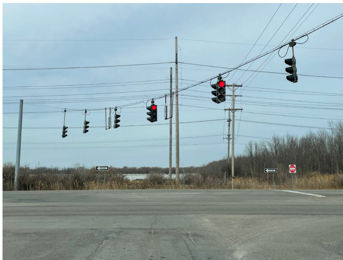
Typical traffic signal installation along NYS Route 104
